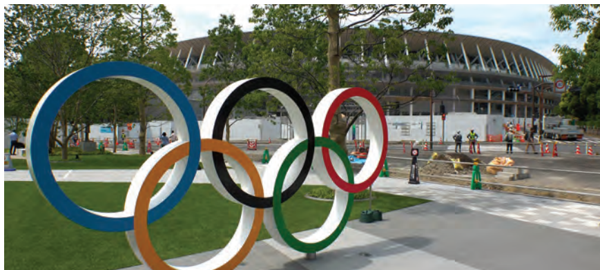
The New National Stadium (pictured) is currently under construction in Kasumigaoka. It will serve as the main stadium for the opening and closing ceremonies
